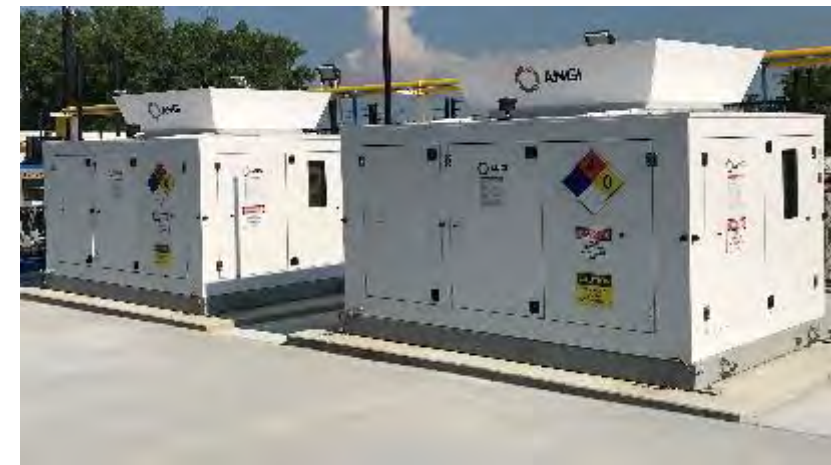
Mother-station loads CNG into Mobile Pipeline® Trailers
