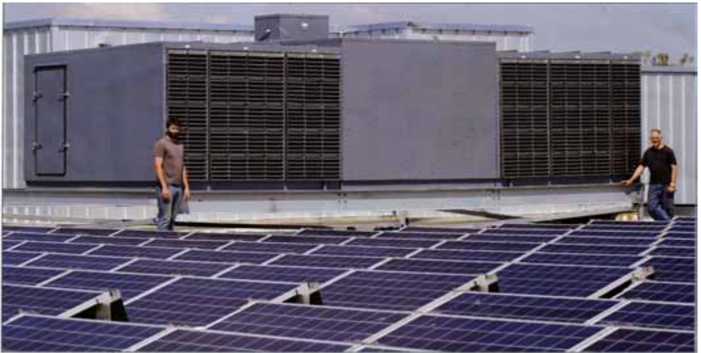
Standing in front of the BKM unit are, left, marketing and sales associate Michael Bullock, and, right, engineering technician Cyril Kuenstler. The unit has ninety 110-pound cassettes, 45 on exhaust and 45 on intake.
