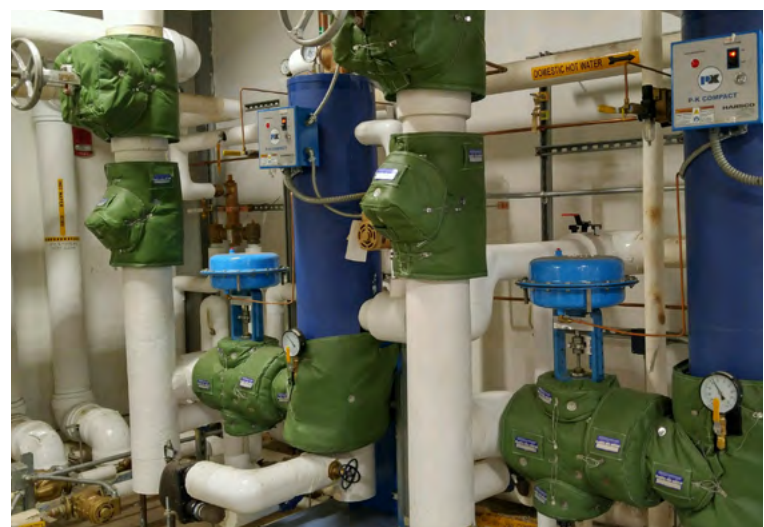
STEAM TO HOT WATER HEAT EXCHANGER Design: LT450TT-1 ½" Thickness Fastener: Stainless Steel Wiretwists / Velcro® Flaps
