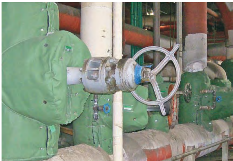
BOILER ROOM – MAIN HP STEAM HEADER GATE VALVES & VALVE BONNETS Design: LT450TT - 1.5" thickness Fastener: Stainless Steel Wiretwists and Velcro® Flaps
