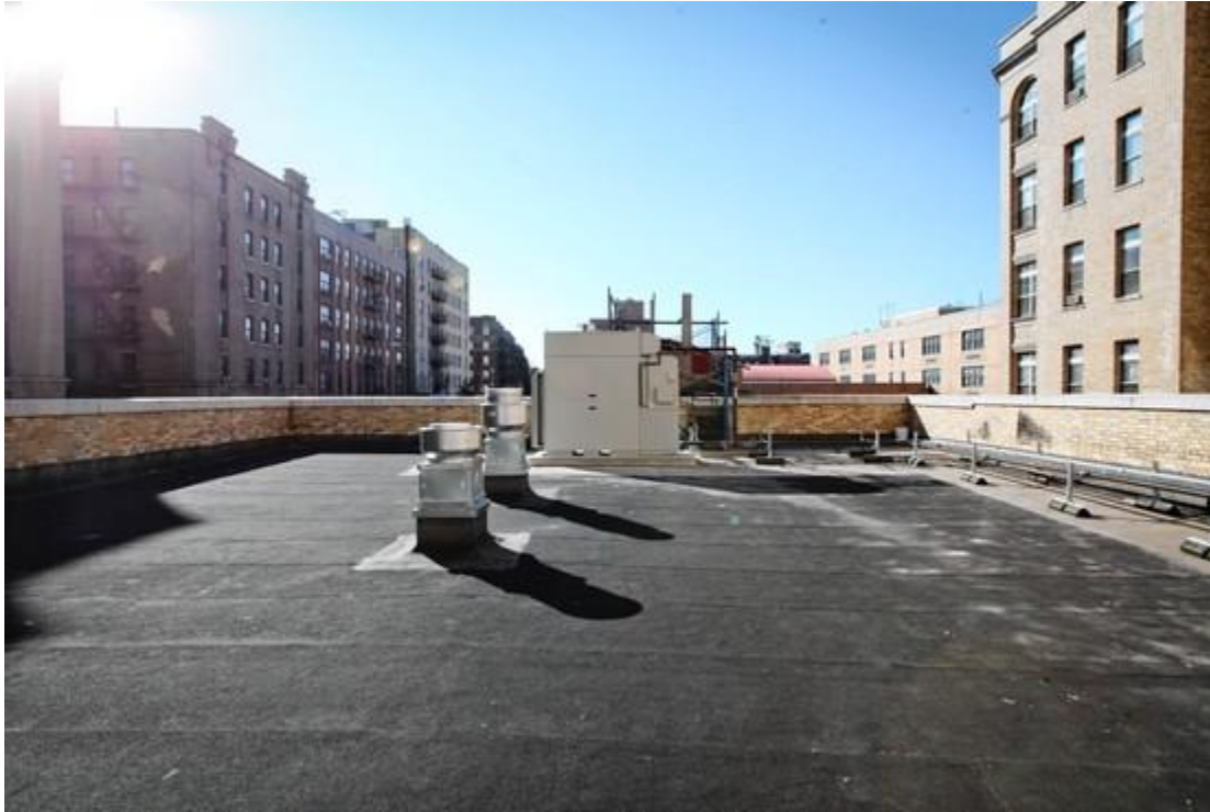
A rooftop 'combined heat and power' unit. Daniella Zalcmán for The Wall Street Journal
