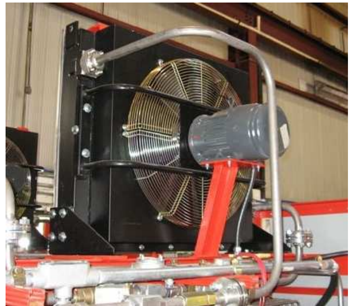
Air Cooled Lube Oil Cooler
