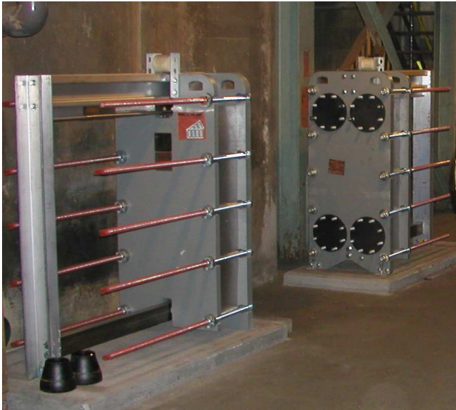
Duplex Plate & Frame Lube Oil Coolers before piping
