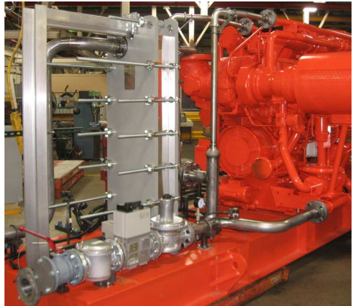
Emergency Power Lube Oil Cooler
