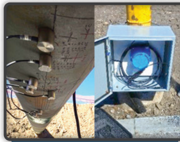
Buried probes attached to pipe and connected to a smartPIMS® Modbus DSI in an above-ground enclosure.
