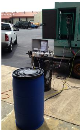
External Fuel Tank
