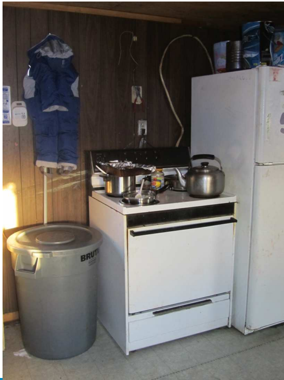
Cooking stove with no range exhaust
