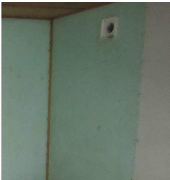
Ventilation intake plugged with a rag
