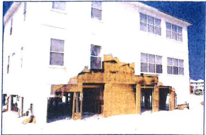
Siding on the non-breakaway portions of this elevated building was extended over breakaway enclosure walls and was damaged when breakaway walls failed under flood forces.
