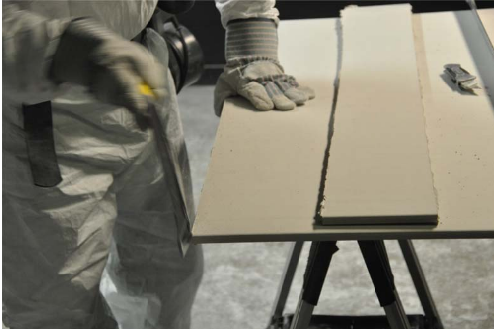
Figure 6. R rasping the rough cut edge of the main drywall board section using the shaping file/forming plane.
