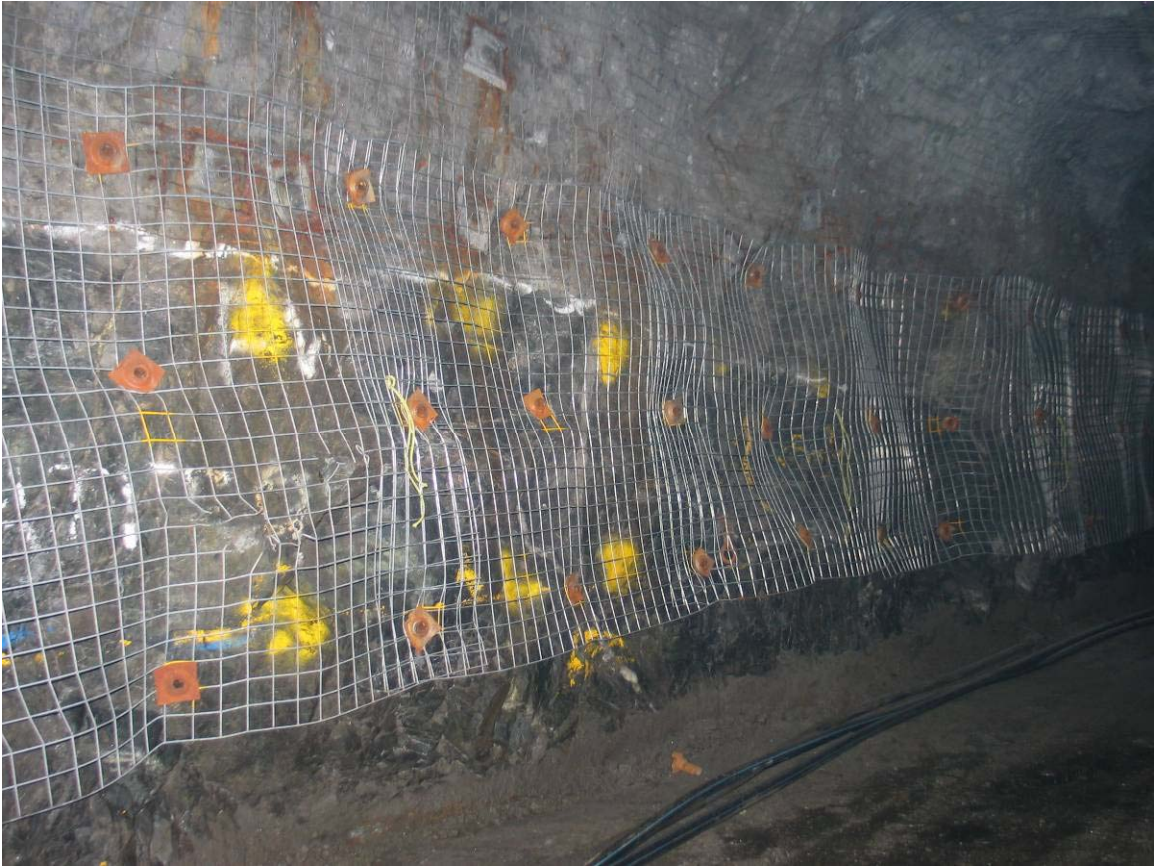
Figure 9: Preparation of the up dip wall, ready for shotcreting at the 465 drive.
