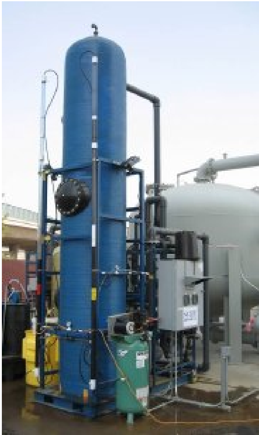
Figure 4: SMI-III ® media column investigation photographs
