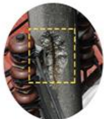
Crack On Pole
