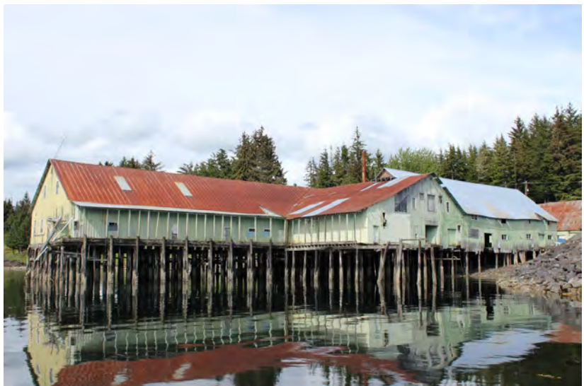
The Keku Cannery now shows signs of deterioration. Stabilization has been started.
