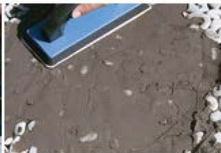
Apply a sanded grout on 2" x 2" sections at a time until the entire installation is covered.
