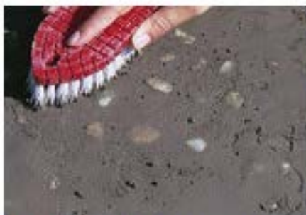
When grout has dried for 30 minutes use a stiff bristled brush to remove the excess grout.
