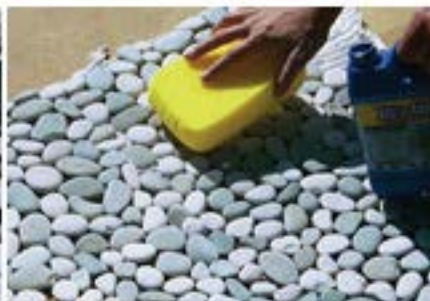
Seal the tiles with a good quality penetrating sealer. Color and shine enhancers can also be applied to vary the finish of the pebbles.
