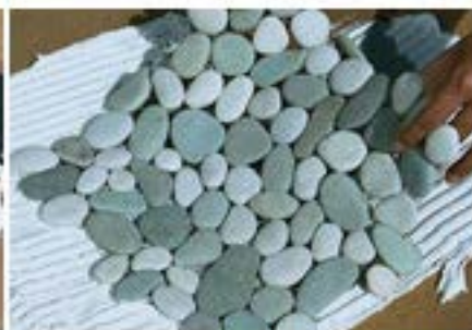
Place tiles on the thinset. Take extra care to get each tile close together using their interlocking shape.
