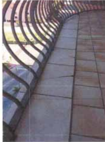
Figure B: Damaged balcony tile that must be removed to fix structural damage
