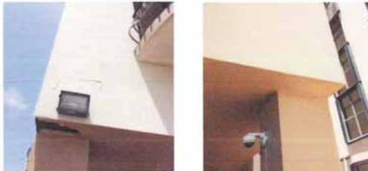
Figure G: Typical cracking in the stucco exterior façade.
