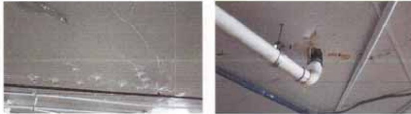
Figure K1: Previously installed failed injection repairs with leaching forming
