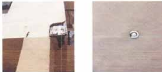
Figure E: Deteriorated plywood soffit above entrance drive.
