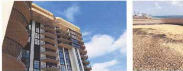
Figure H: No suspension hooks at the underside of the balconies and on the roof.
