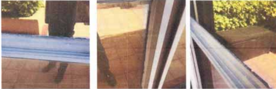
Figure F: Exterior sealant at window frame that has aged past its serviceable lifespan
