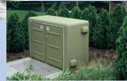
A packaged submersible pumping system is used to transfer sewage to a treatment facility.
