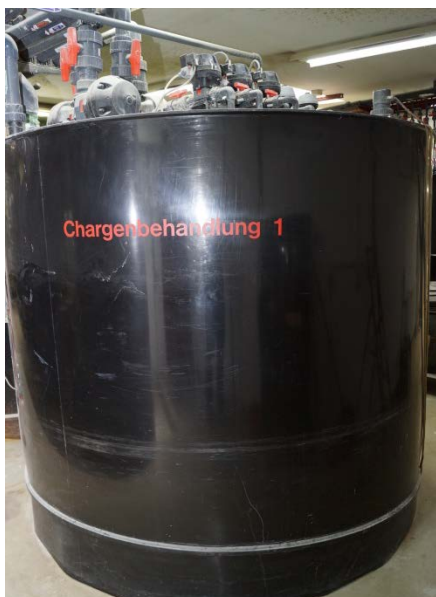
Photograph shows wastewater holding tank.
