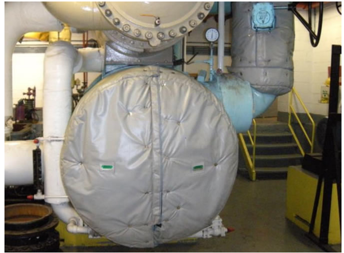
Liquid Chiller Water Box & Control Valve
