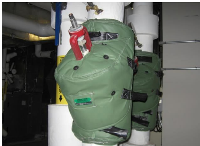
3" 150# "Hot Water" Control Valve
