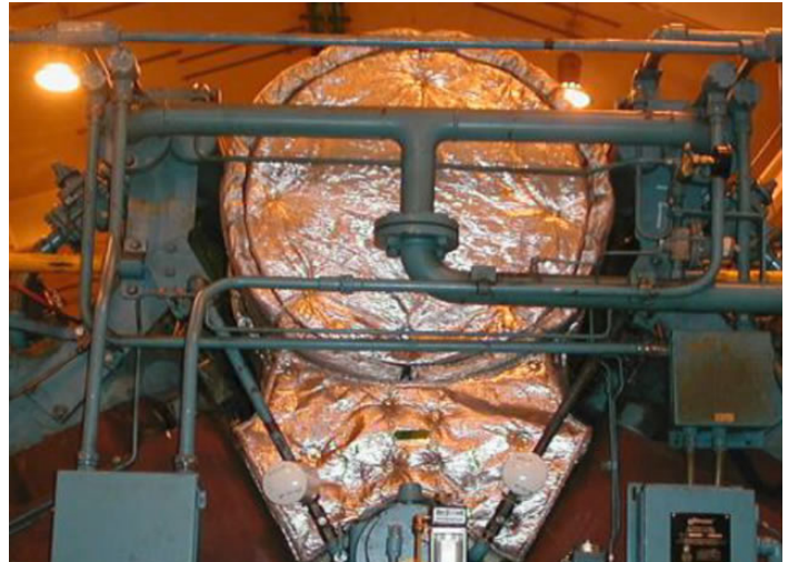
Cooper Bessemer Engine Exhaust Manifold, 2" Thickness
