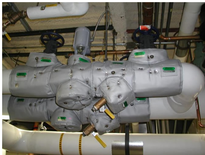
Gate Valve, Strainer, Control Valve, Gate Valve Steam Fitting Assembly
