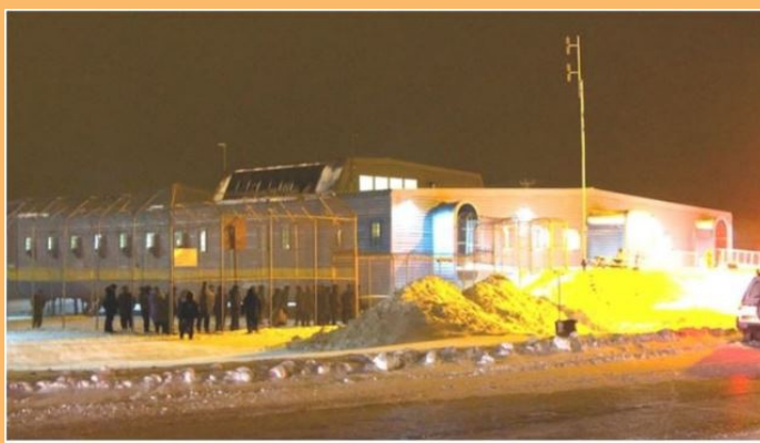
The battered building known unaffectionately as BCC reveals why, in 2013, a federal investigator said it was unsafe for inmates and staff. (Vincent Desrosiers/CBC)
