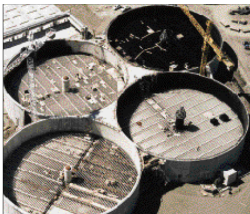
Four trickling filters, part of the world's largest trickling filter/solids contact system, are shown during construction.
