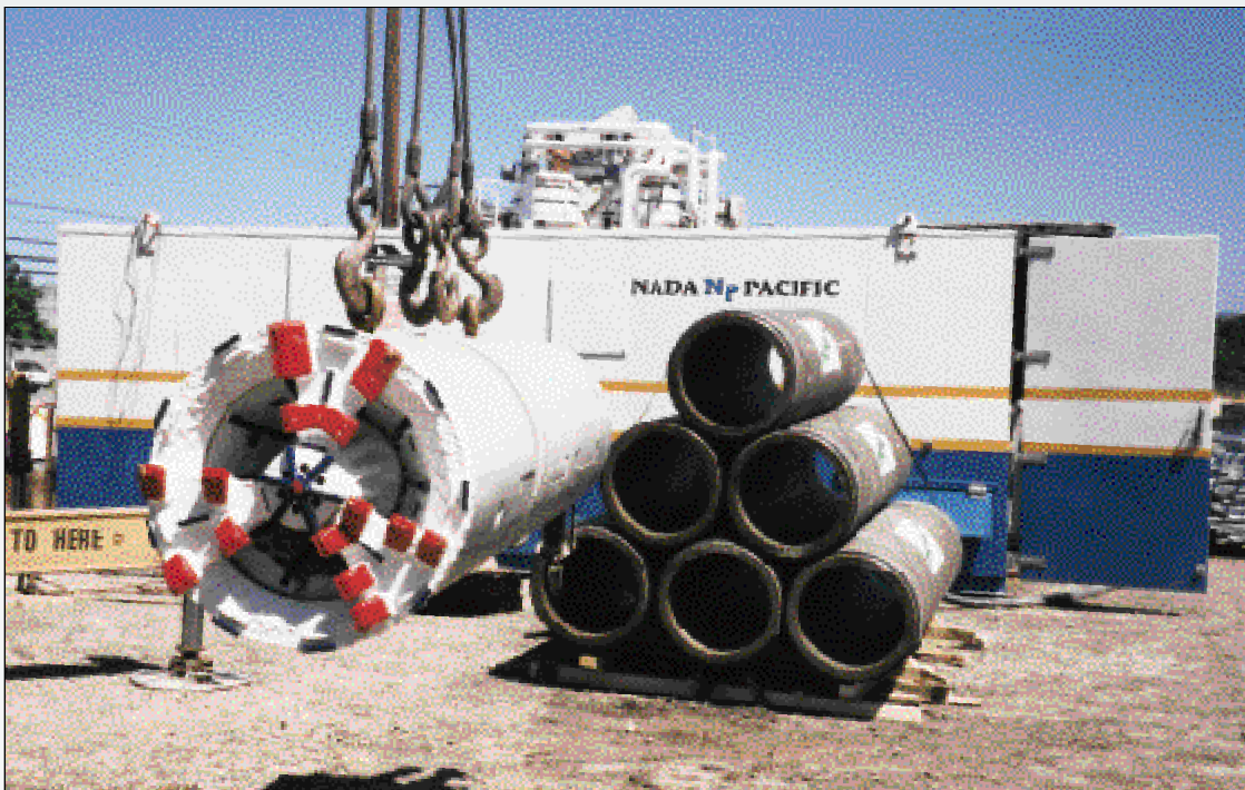
To install more than 5,000 feet of new sewer main along a busy street in Fremont, Calif., Brown and Caldwell recommended microtunneling. Shown are the tunnel-boring machine and the pipeline before installation.
