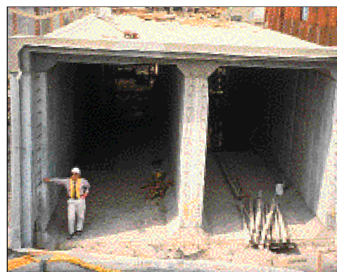
Brown and Caldwell/ABR project manager Steve Krugel stands in the Annacis Island facility's secondary effluent conduit, now completely operational beneath the ground surface.
