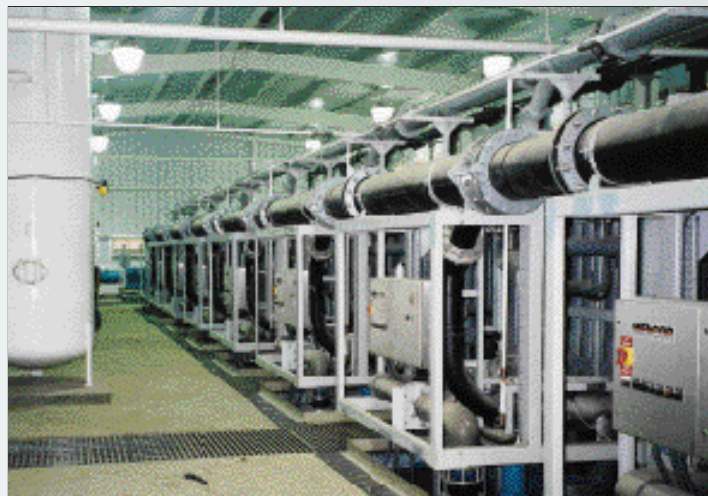
The eight microfiltration membrane units at the Kamole Weir Water Treatment Facility, Maui.
