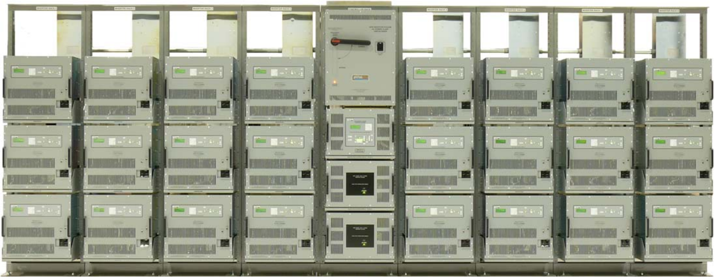
Inverter System as shown above: 180 kVA / 168 kW 3 Phase N+1 Redundant
