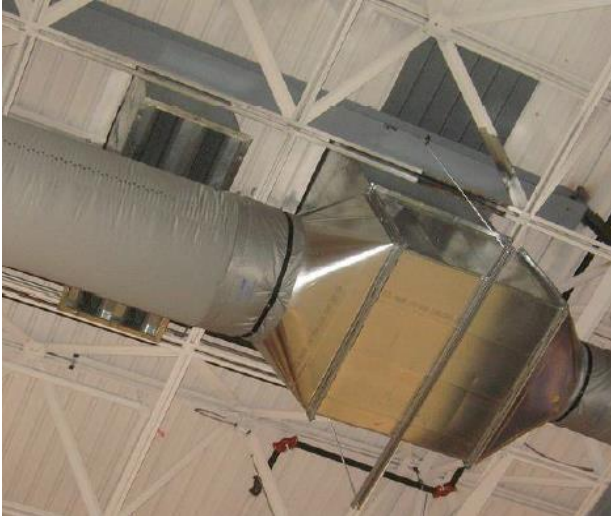
Whisper™ “V” System with vertical silencers (below deck view – open return)
