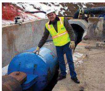
In Memoriam: Steve McCandless The project team would like to recognize Steve McCandless of Garney Construction, who passed away shortly after completion of the tunnel lining. His colleagues saw Steve as incredible person in every way and an inspiration to many.
