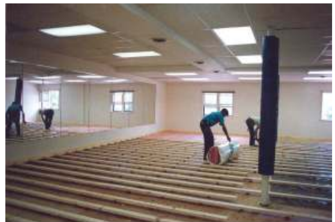
Second floor karate studio isolated from retail store below using type WFF Wood Floating Floor system (see detail at left).
